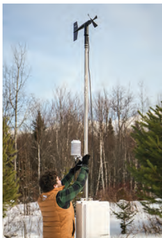
Mesonet and Information Systems Technician Colby Morris and Keith Garrett, MWOBS Director of Technology, install a remote weather station near the recently installed LiDAR unit.
